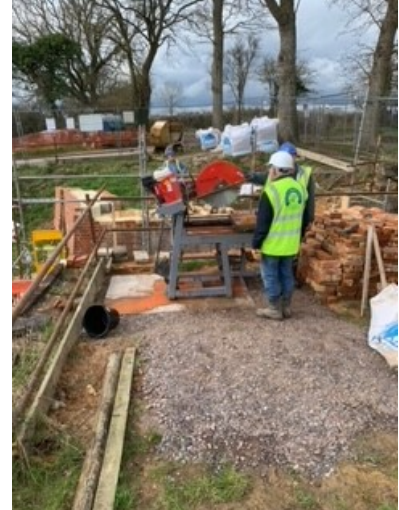
the bench saw plinth in place (top) and the bench saw positioned
